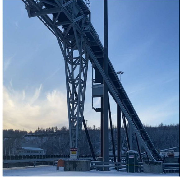
4. Elevated Conveyor feeding Ship Loader
