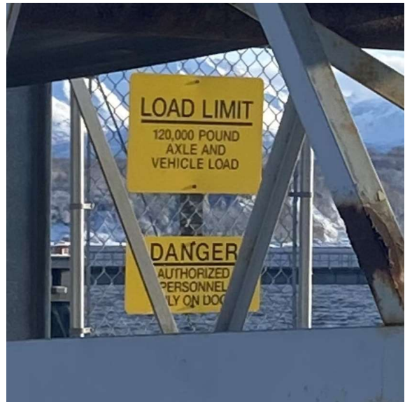
2. Load Limit Sign on Trestle
